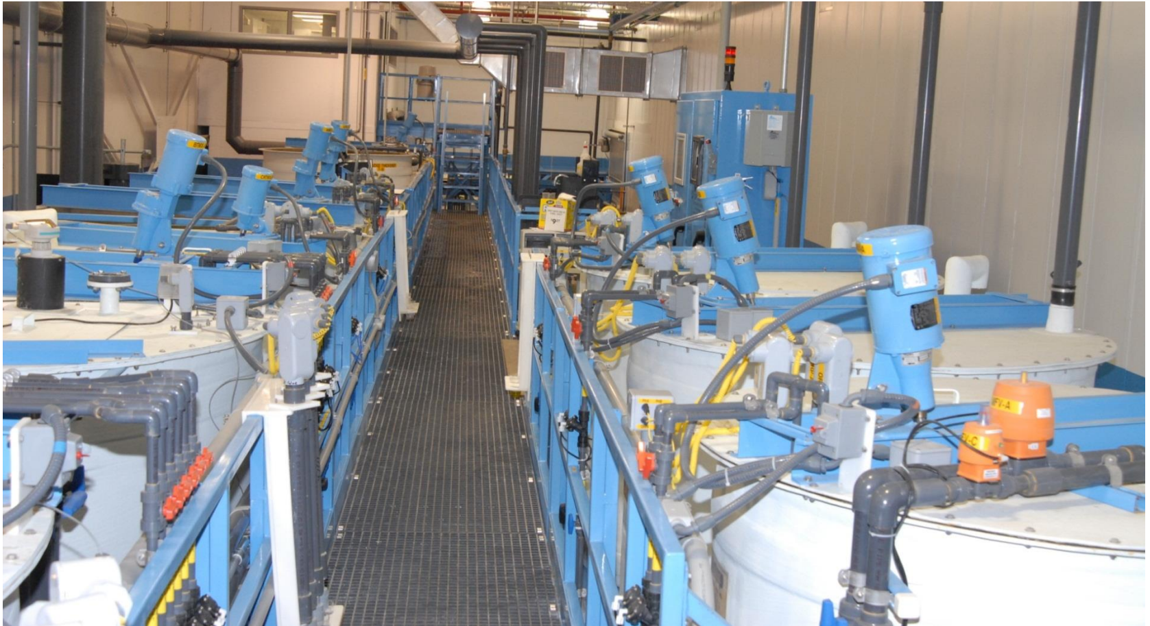
90 gpm Chrome and Cyanide Treatment System for the job shop plater
