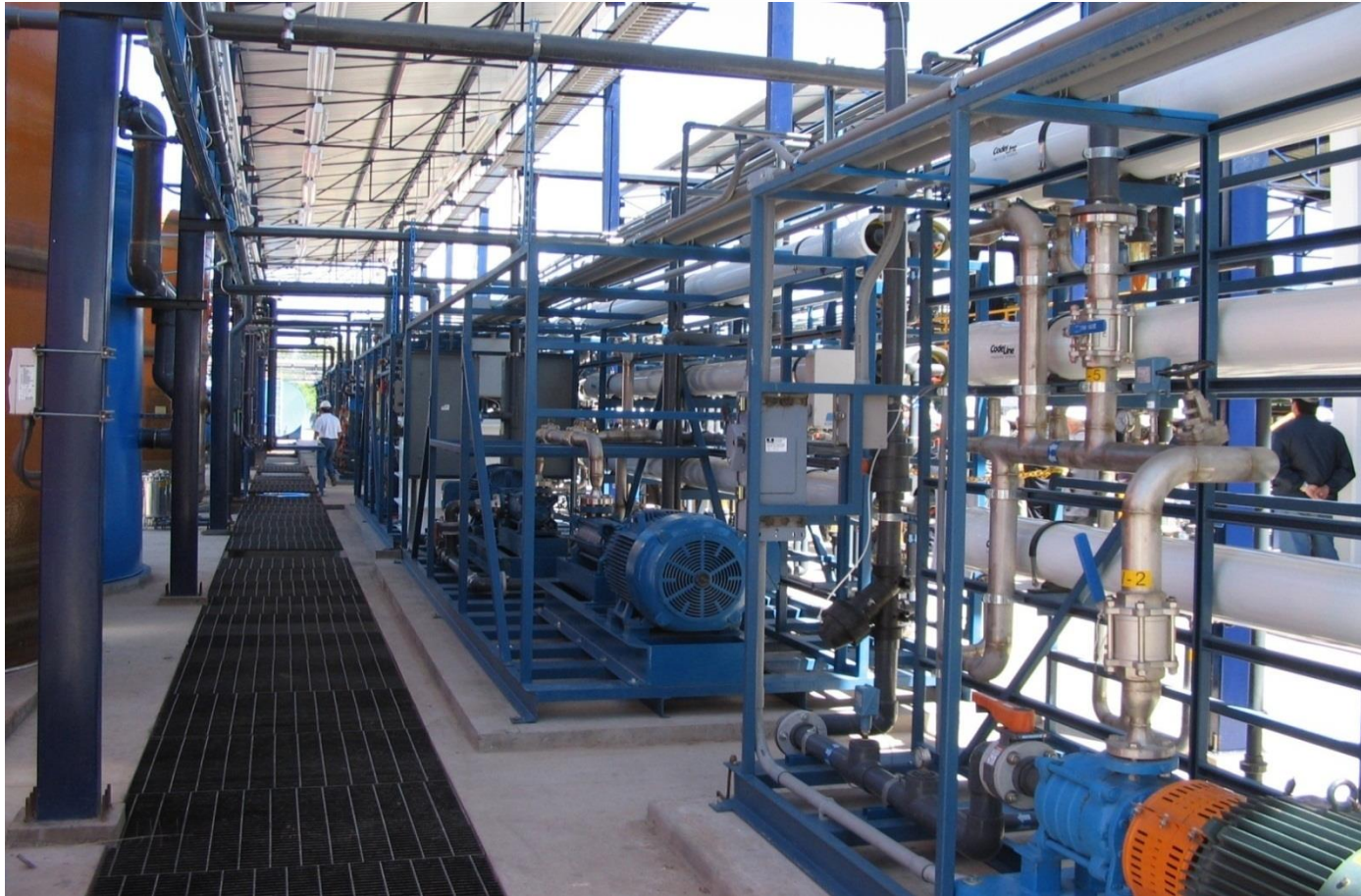
3 RO Systems for Water Recovery/Recycle at 225 gpm
