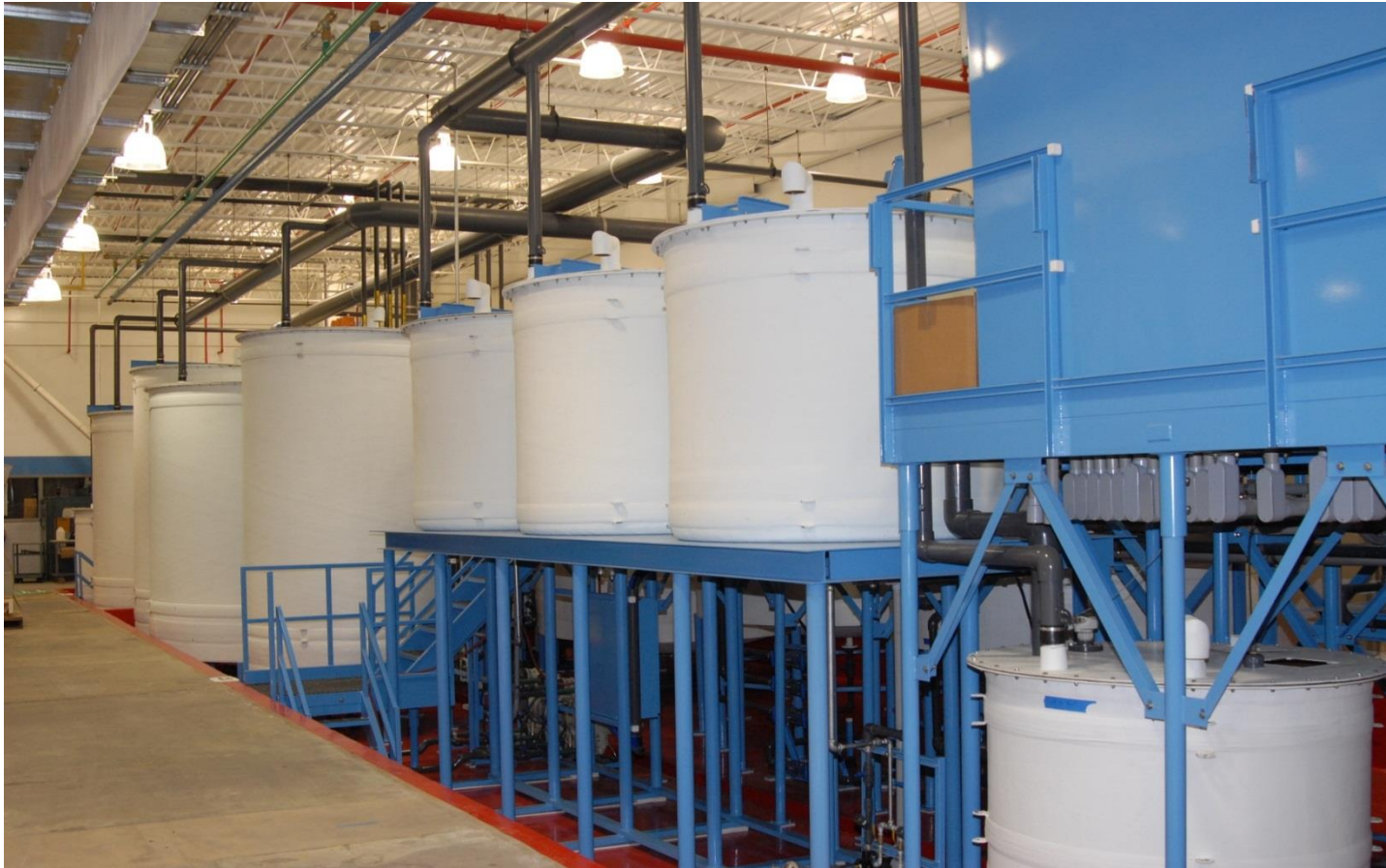
90 gpm Treatment System with custom colored fiberglass tanks for the job shop plater
