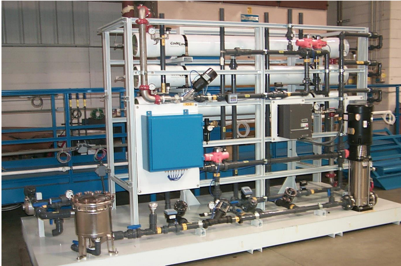
15 gpm fully automatic RO for Water Recovery
