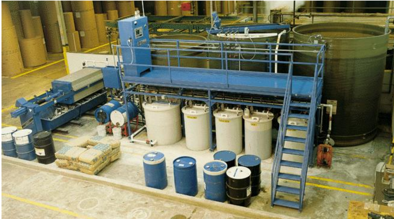
Batch Treatment 5000 Gallon Capacity
