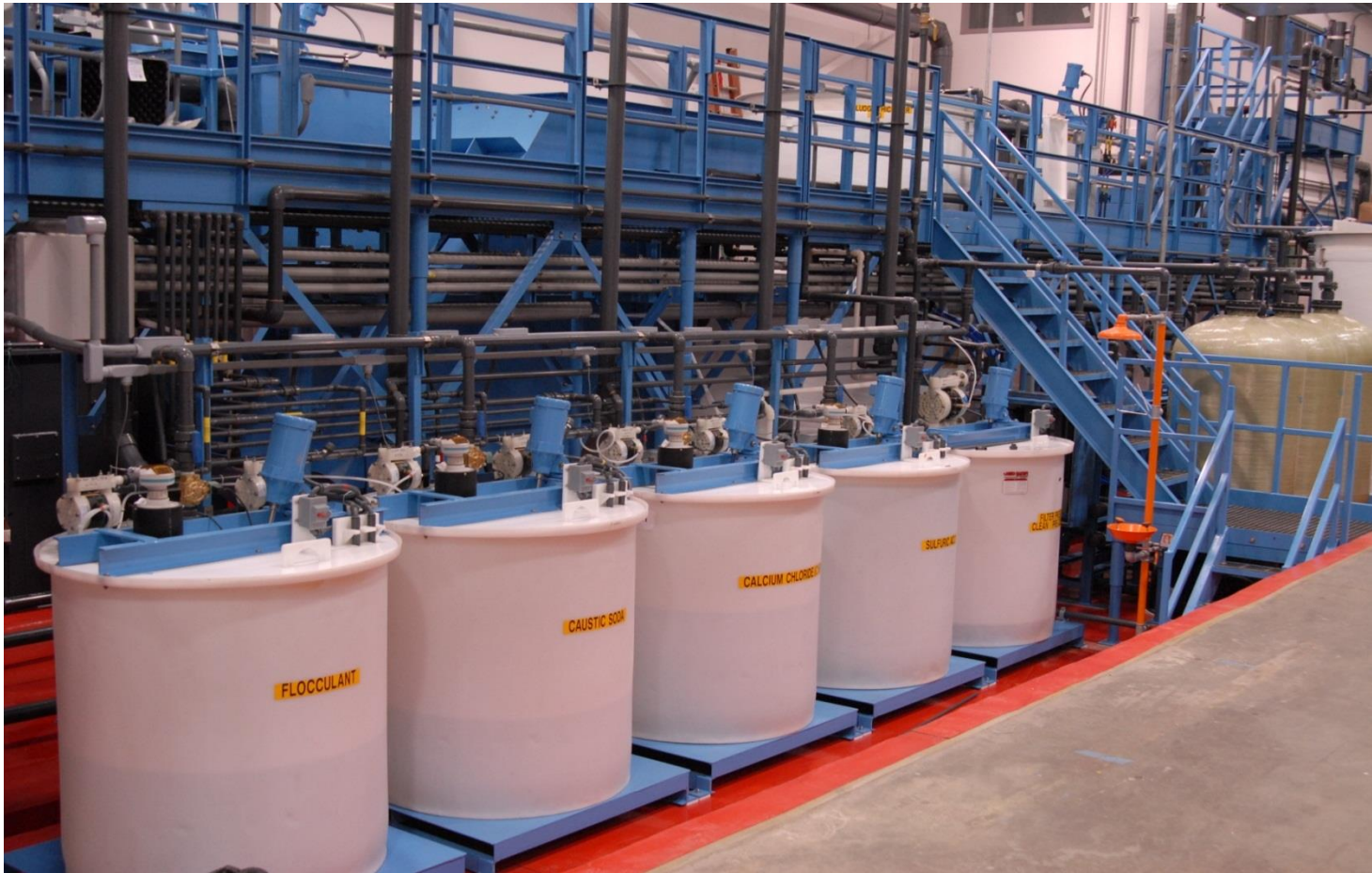
Chemical feed system with automatic make up for the job shop plater
